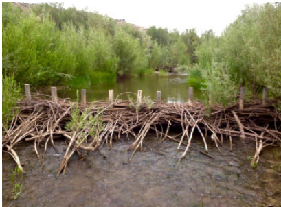
In Oregon's Bridge Creek Watershed, researchers built a number of beaver dam analogs to encourage increased beaver activity and restore river habitat. Credit, Utah State University
