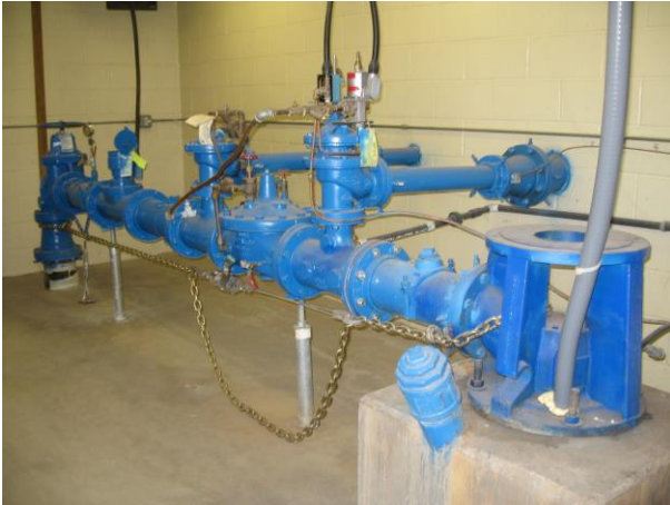
Photo 1 – Barney Well and piping.
