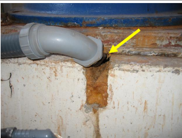
Photo 8 – Seal around power cable going into 4 th Street Deep Well.
