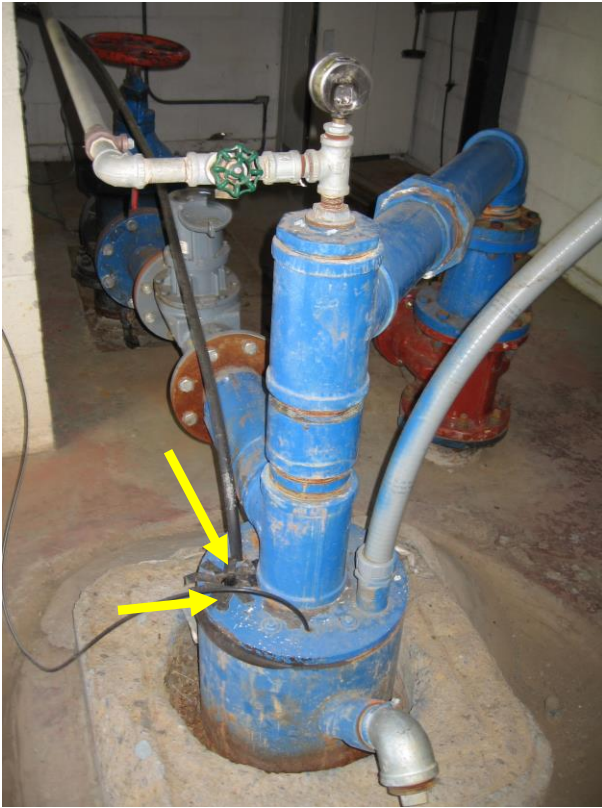
Photo 12 – Ochoco Heights Well is not used. Seal openings on wellhead. Source should be disconnected from distribution as a protective measure.
