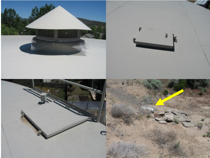
Photo 23 – American Pines Reservoir protected overflow pipe, locked curbed hatches and screened vent.
