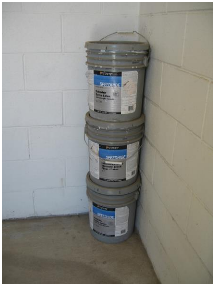
Photo 20 – Remove paint stored in Airport Well 2, Lamonta Well and Ochoco Heights Well buildings.
