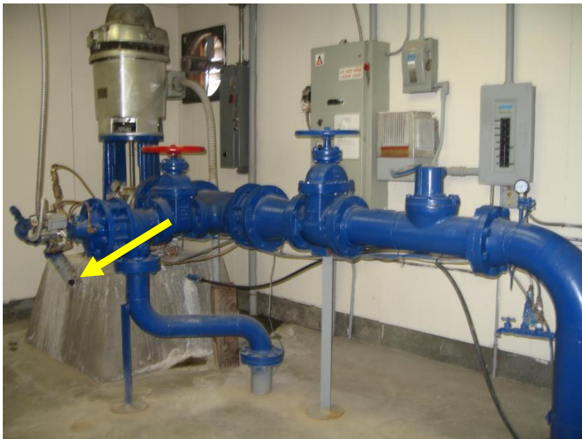
Photo 24 – Seal opening into concrete pad for Stearns Well (covered with black tape).
