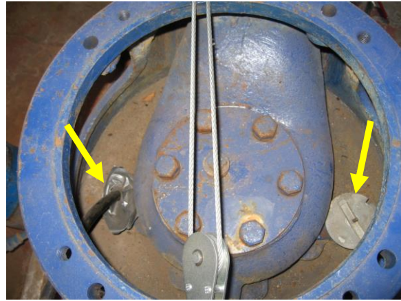
Photo 9 – Seal down-hole chlorine opening into 4 th Street Deep Well (under duct tape). Improve cover to hole for measuring water level.
