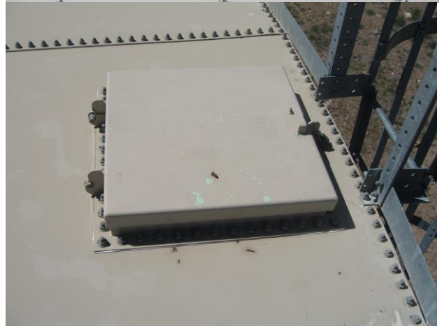
Photo 22 – Airport Reservoir protected overflow pipe (arrow), locked curbed hatch and screened vent.
