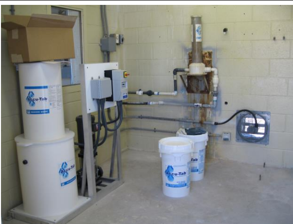
Photo 3 – New chlorination equipment for Barney Well.
