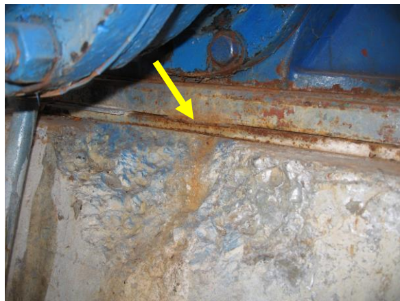
Photo 10 – Seal gap between pump platform and concrete pad on 4 th Street Deep Well.
