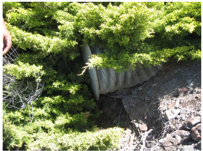
Photo 14 – Remove vegetation away from overflow pipe/valve for Ochoco Heights Reservoirs.
