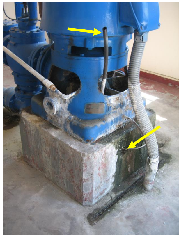
Photo 15 – Seal opening on well with tubing and hole in concrete pad for Yancey Well.
