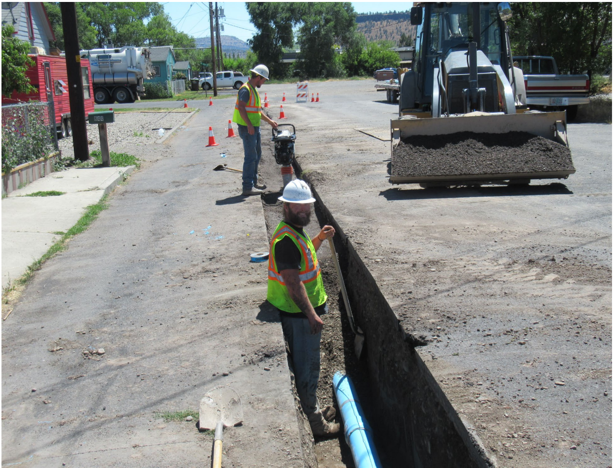
Public Works crew members working a water line at NE 6 th and NE Belknap Streets in September 2020
