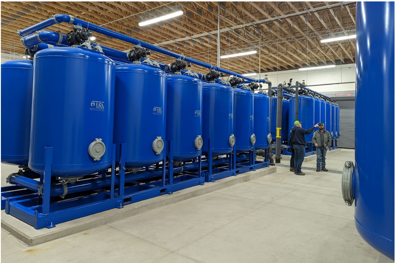
The new water treatment plant facility, part of the ASR project, in December 2021
