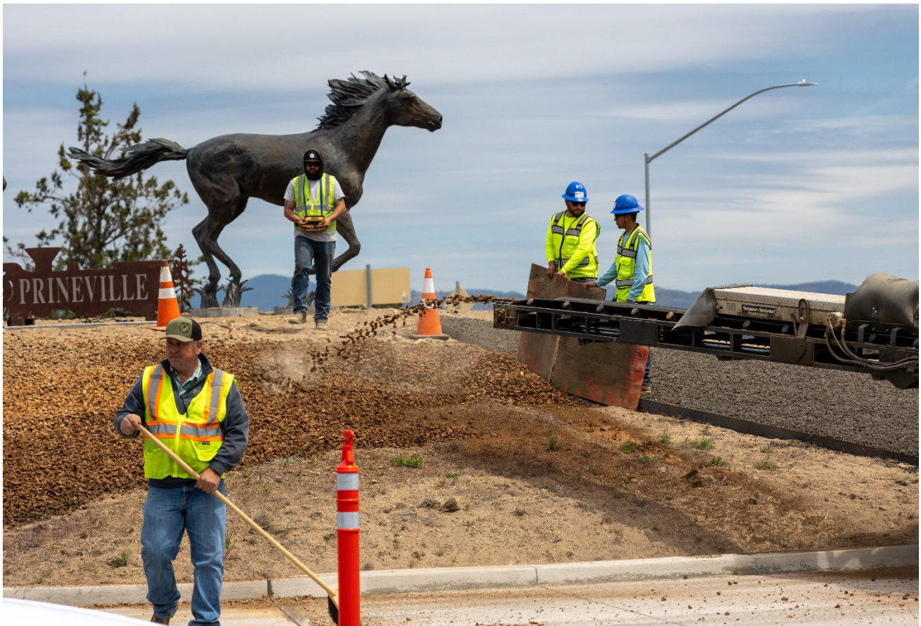
Street Superintendent Justin Severance (far left) working on the Tom McCall roundabout project in July 2022
