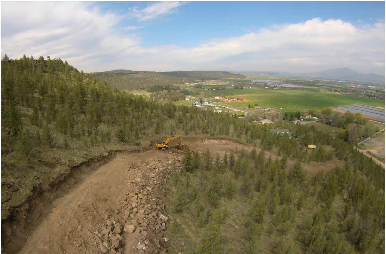
Beginning construction phase of installing new utility lines to connect the airport industrial area to the valley floor in 2018
