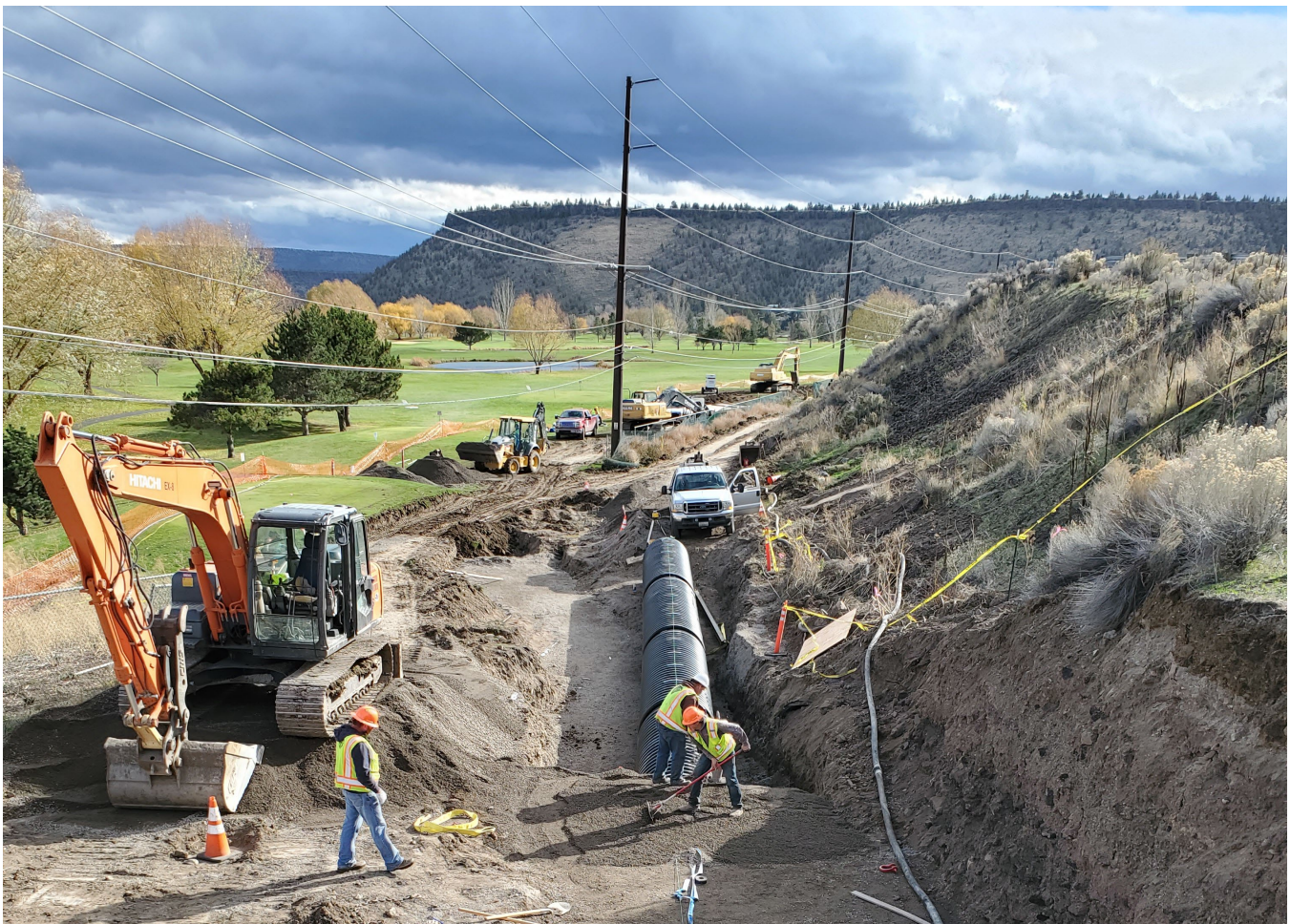
Public Works worked with a local contractor in 2021 to replace a Peoples Irrigation District pipe next to Meadow Lakes Golf Course
