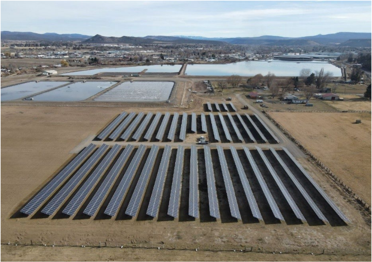
Solar field at the wastewater treatment plant facility
