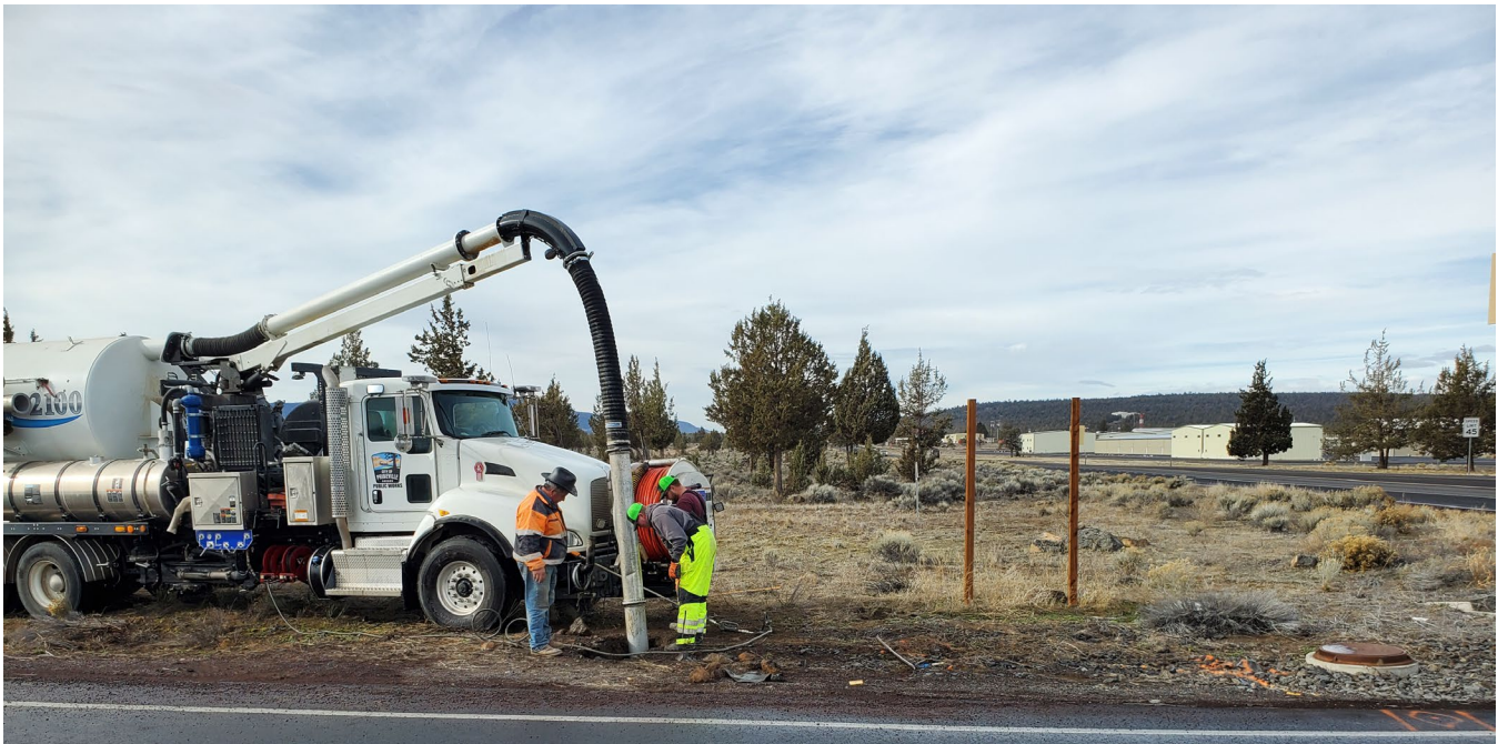
Public works staff working a vacor truck near the Prineville-Crook County Airport in March 2022
