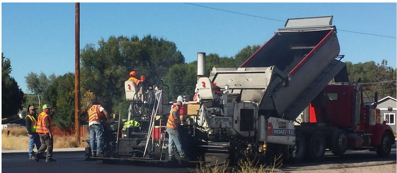
Contractors and City staff lay asphalt during the NE Juniper Street paving in October 2017.
