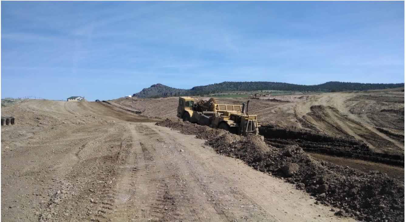
In order to support the newest school in the district, Barnes Butte Elementary, work had to be done to extend streets in 2015.
