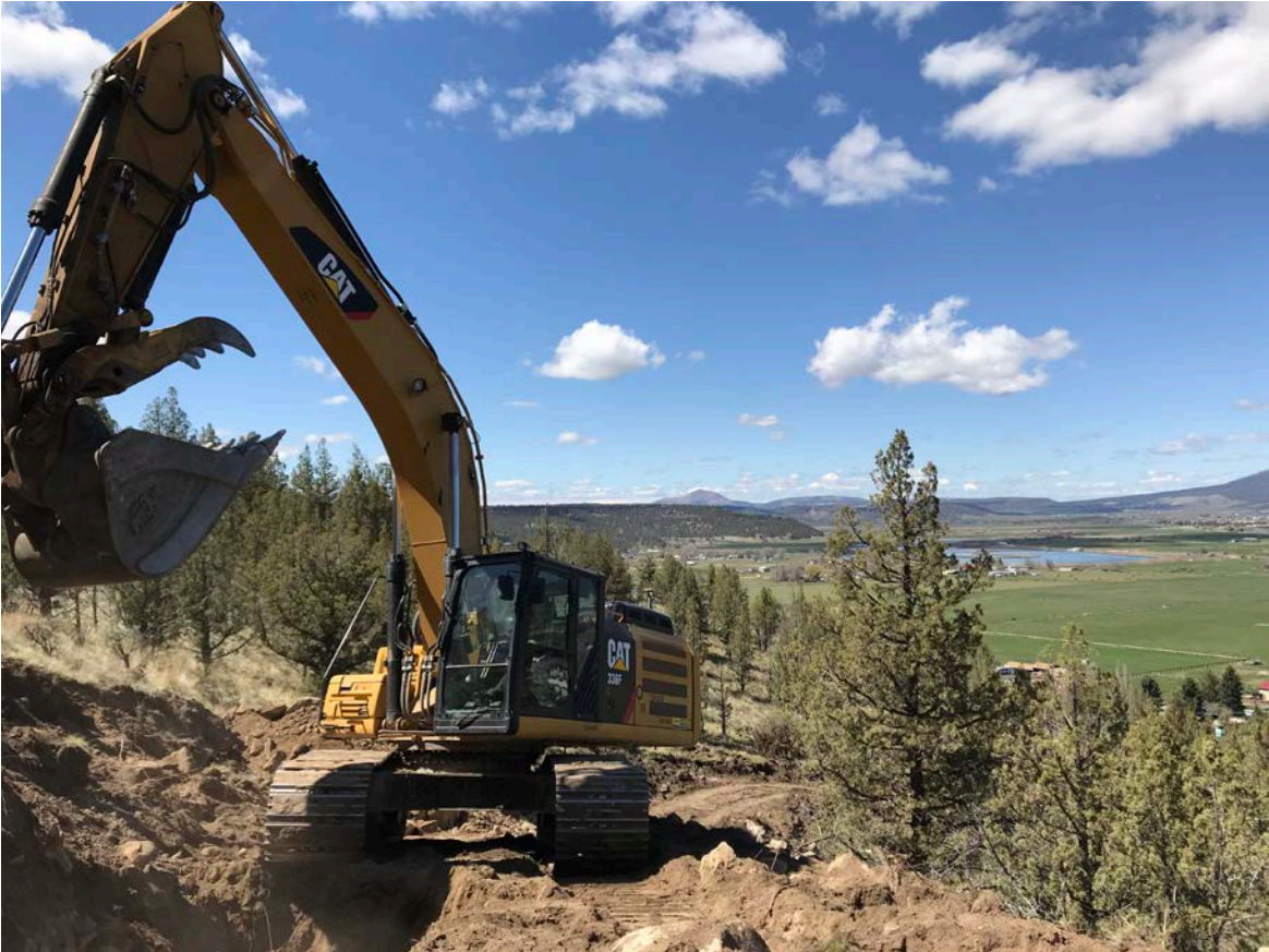
Contractors excavate the hillside as part of the Airport Industrial Park Utility Extension project in April 2018.
