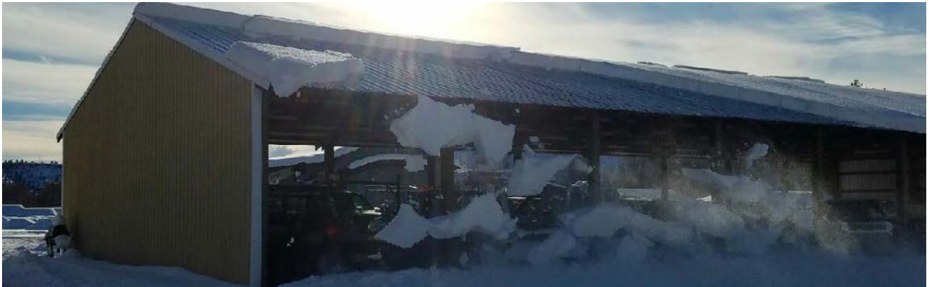
After a heavy snow build up at the Public Works offices in January 2017, sunlight broke to begin winter melt off.
