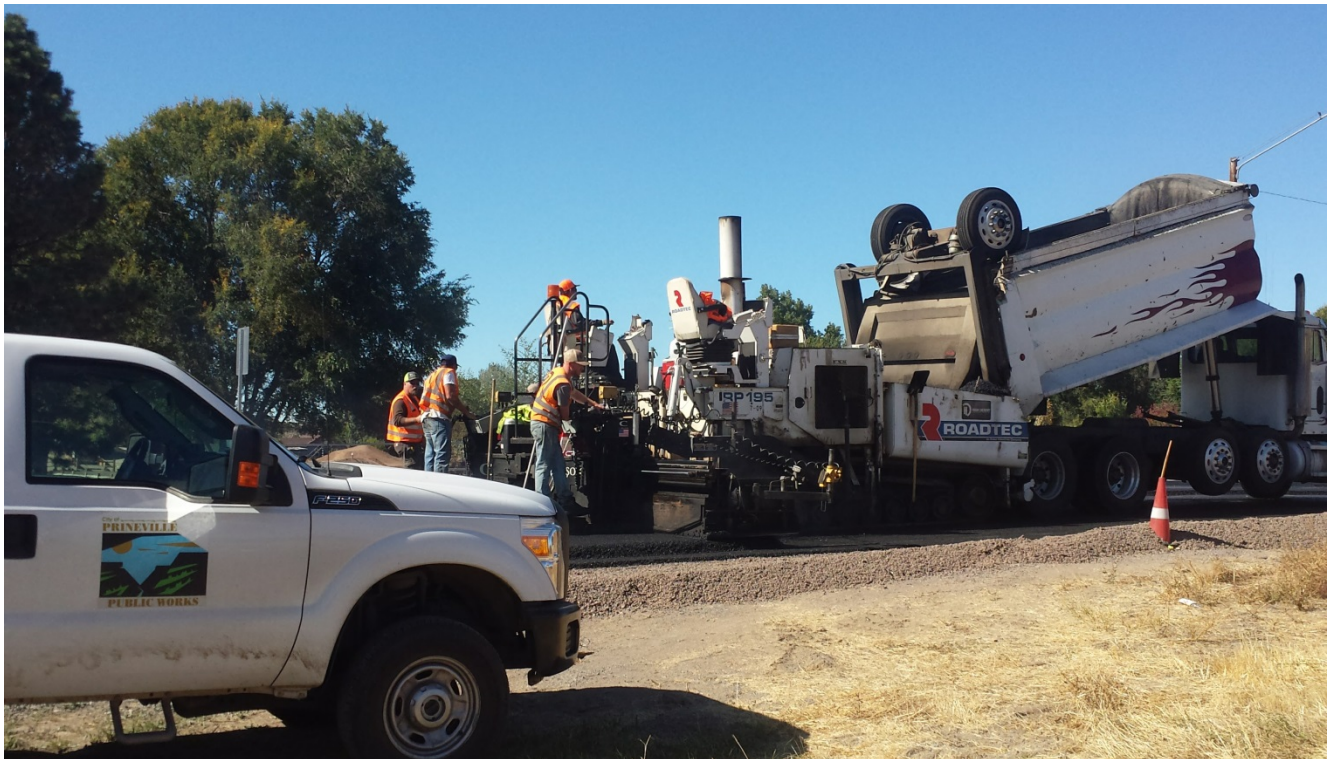
Crews work to lay down asphalt on NE Juniper Street during a paving project in October 2017.
