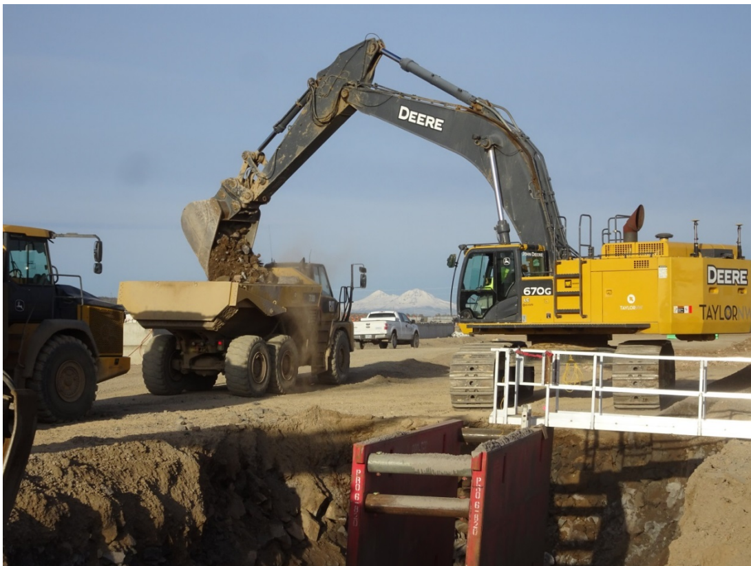
Heavy machines move earth to install a sewer line roughly 28 feet deep near the airport industrial park.
