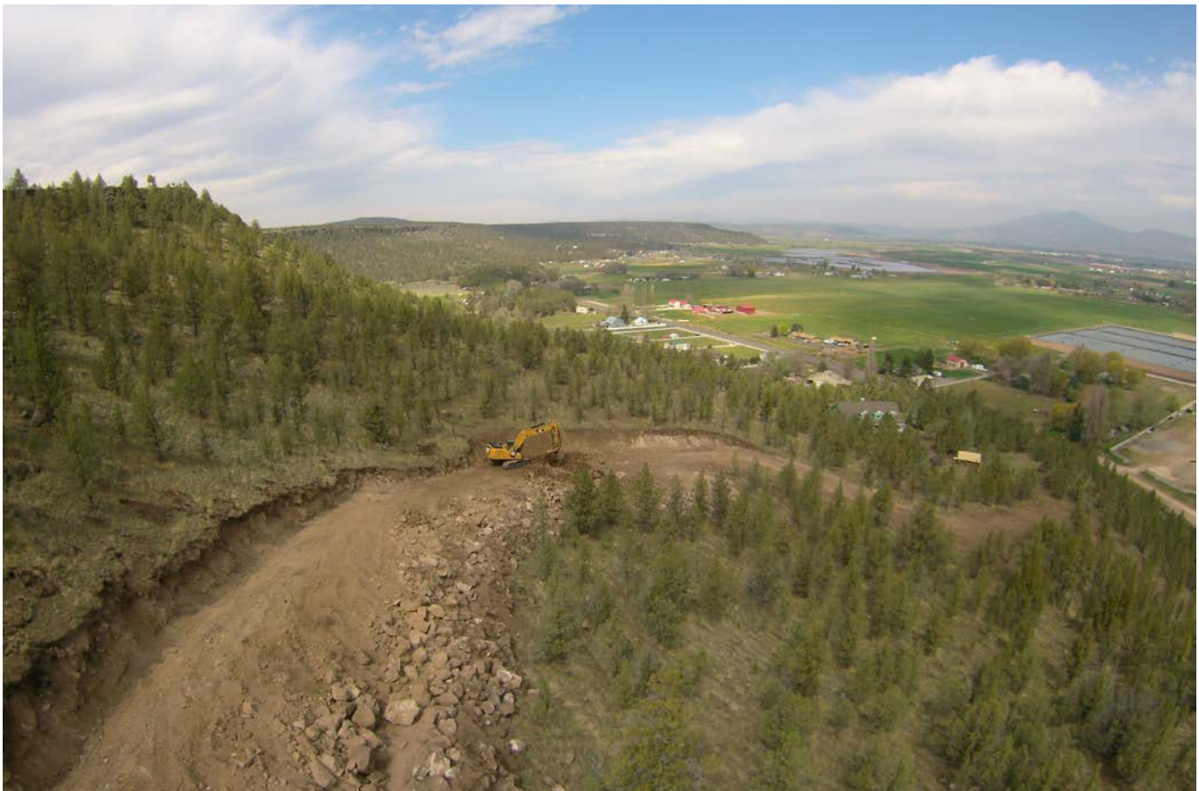
The construction phase to install new utility lines to connect the airport industrial area to the valley floor began in 2018.
