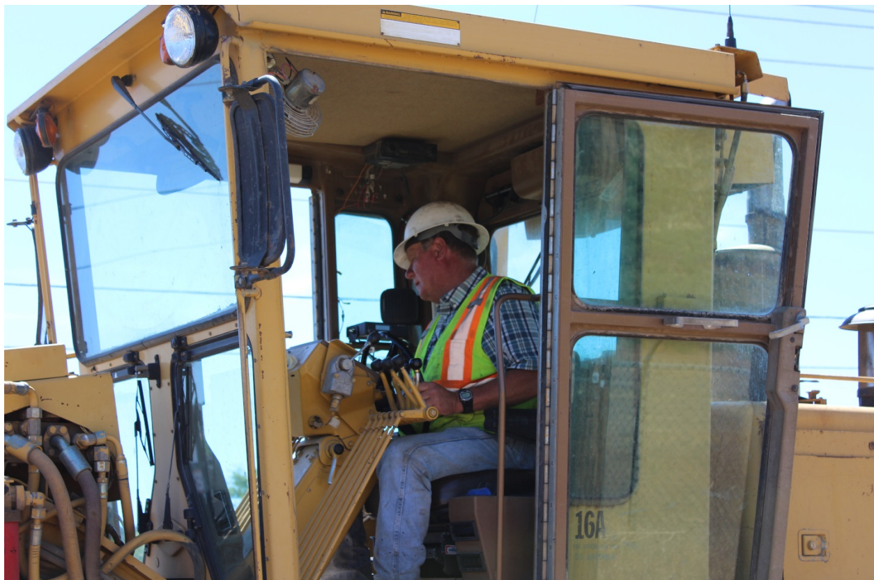
Street Superintendent Scott Smith works a grader during a paving project in June 2017.
