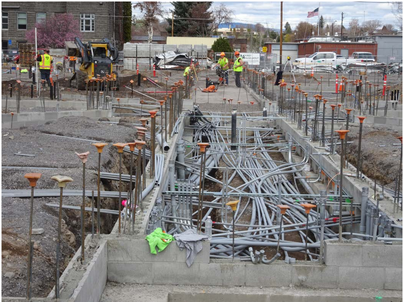
In 2019, the IT Department is working with the Crook County Sheriff's Department on installing technology infrastructure and cameras into the new jail, including wiring through conduit built into the foundation.
