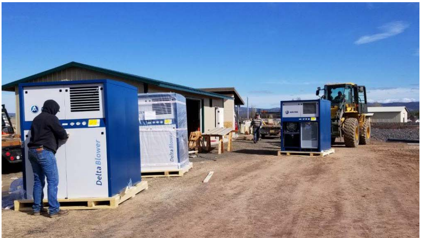
New blowers were installed as part of an aeration upgrade at the wastewater treatment plant in April 2019.
