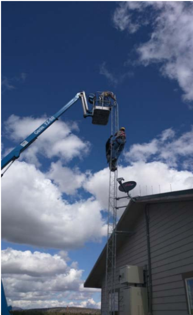
The IT Department works to install cameras at the Prineville-Crook County Airport terminal.
