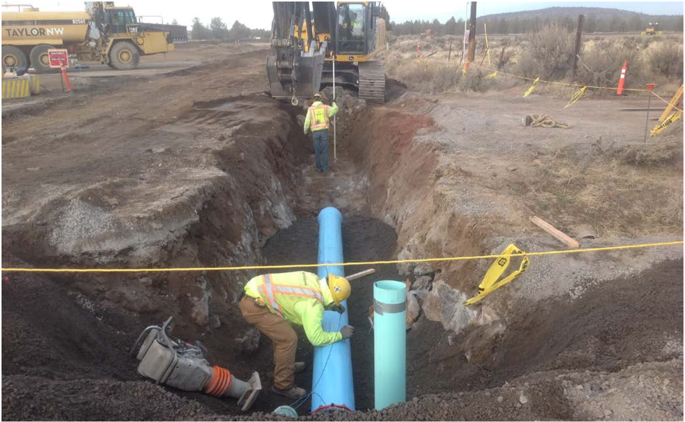
Contractors work to install lines as part of the Airport Industrial Park Utility Extension project in February 2018.
