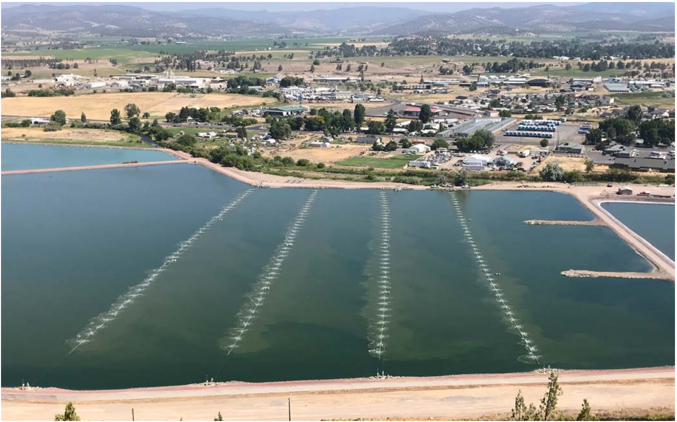
After an aerator upgrade project at the wastewater treatment facility in August 2018, staff captured the system in action from a nearby hill.
