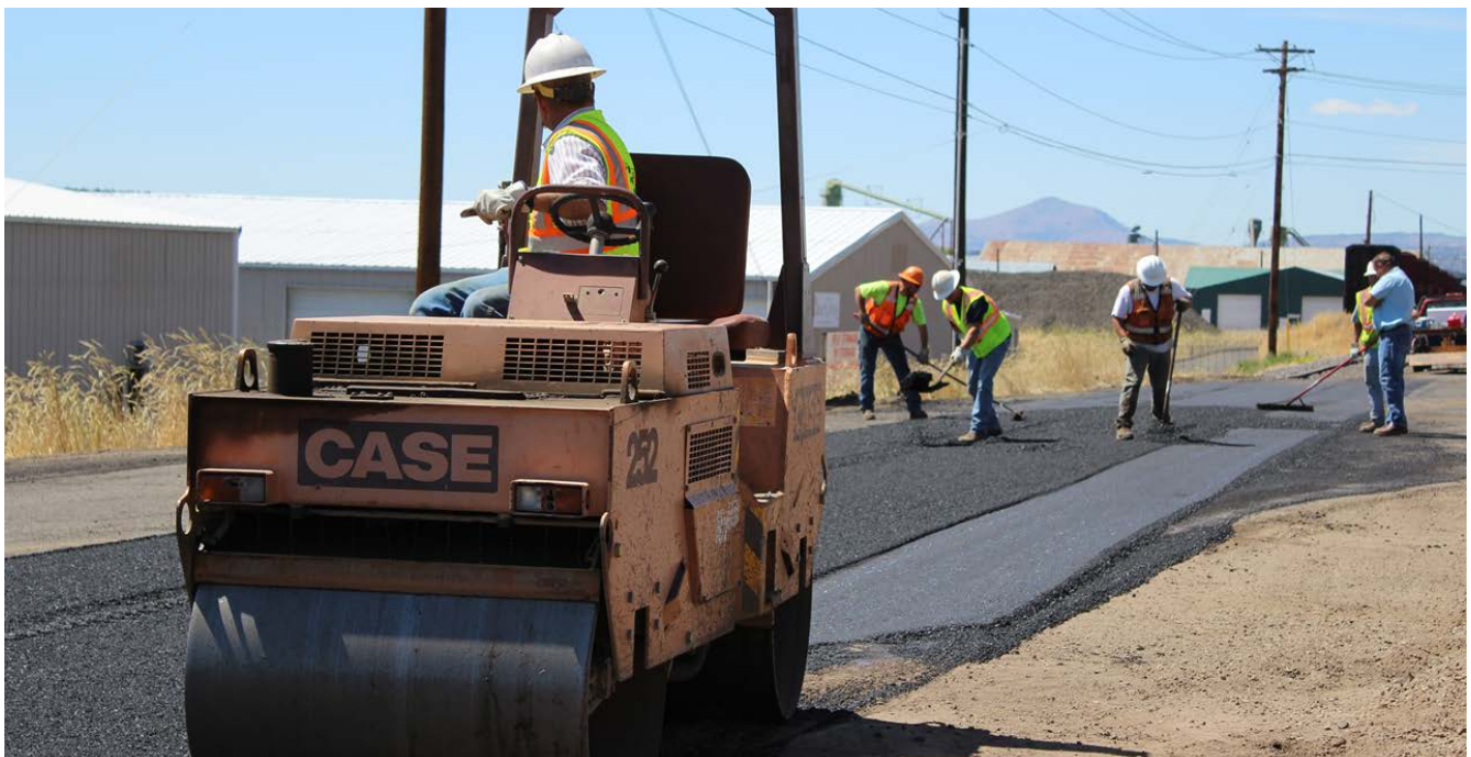
A Public Works crew and contractors work together pave a road on the northwest side of town in June 2017.
