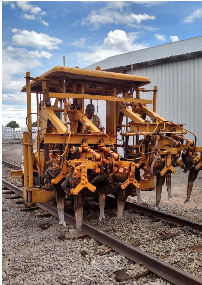
Tamping and leveling a newly constructed yard spur at the Prineville Freight Depot.
