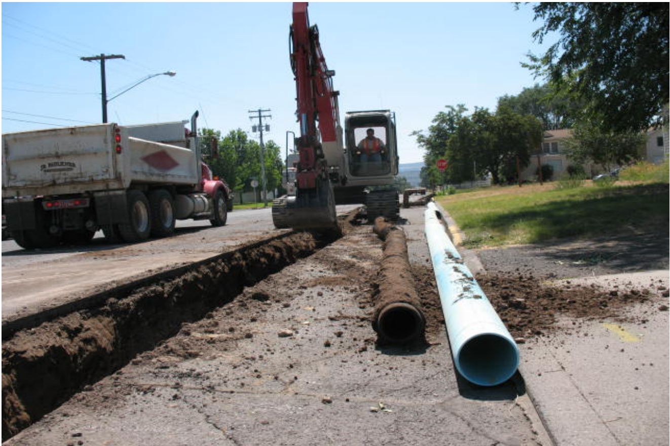
Members of the Public Works Department replace an old, wooden water main with larger plastic lines.
