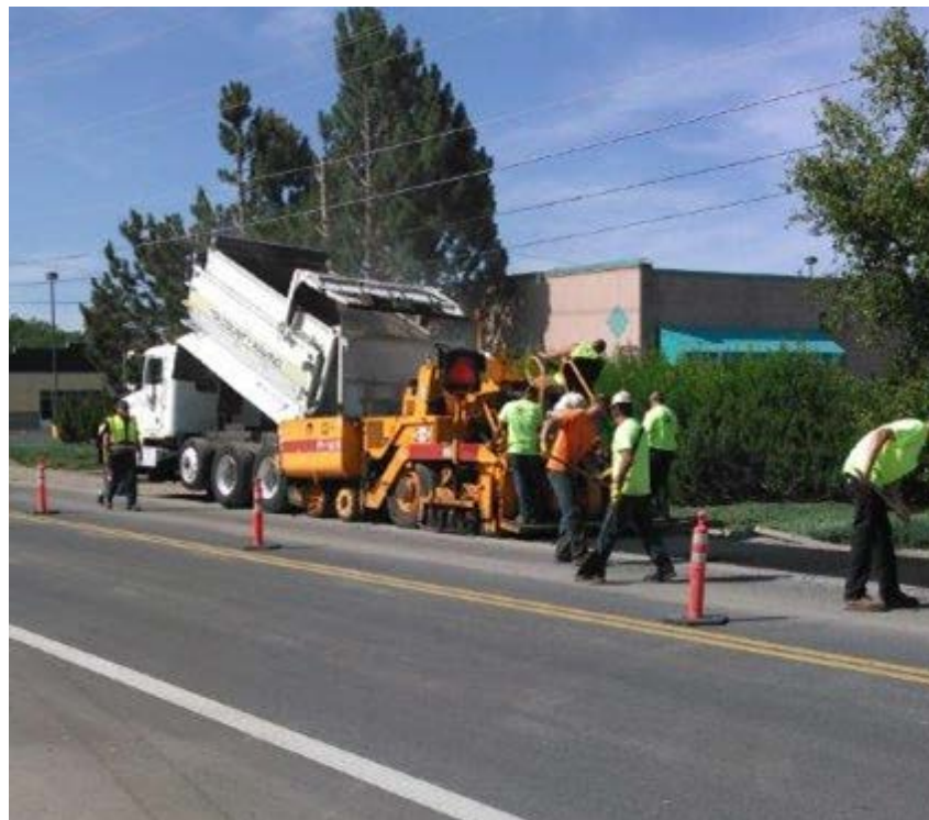
Contractors work on a bike lane infill project on NE Combs Flat.
