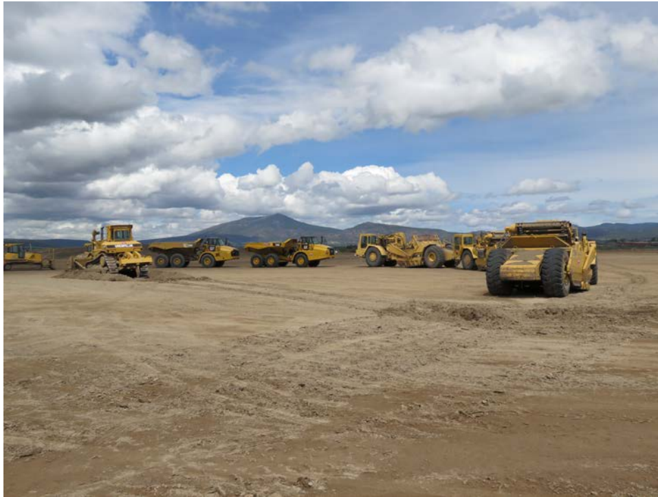
Heavy machines circle up for the Crooked River Wetlands groundbreaking ceremony in April 2016.
