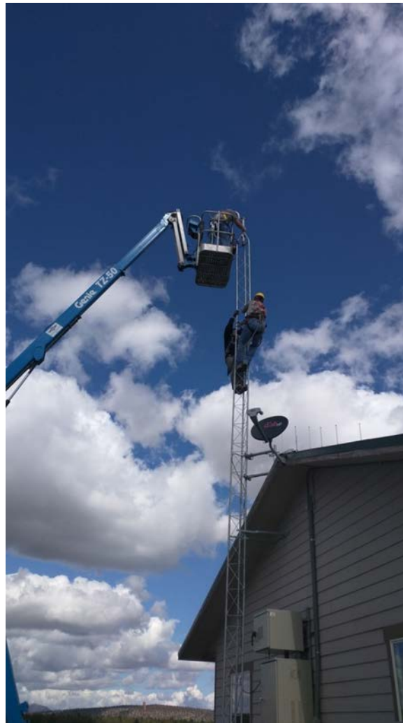
Cameras being installed at the airport terminal by the City of Prineville IT Department.
